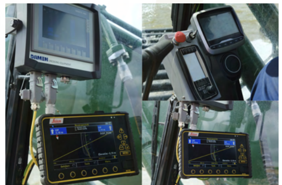
GPS system, powerpack dashboard and DOP pump dashboard
